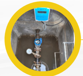
Buan, Jeollabuk-do Direct installation in the hall
