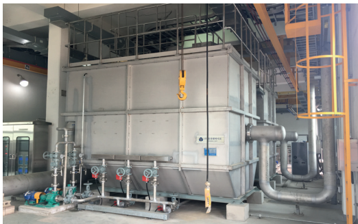
YDFS-2306-1F x 2units Han River water treatment(6,000m 3 /d)
