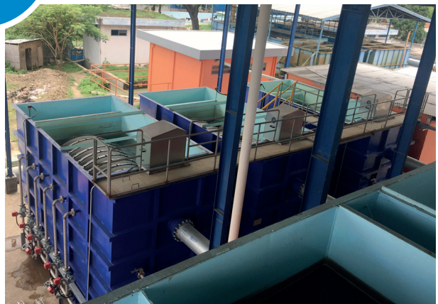
>> Babelan Purification plant, Indonesia(38,880 m 3 /d)
